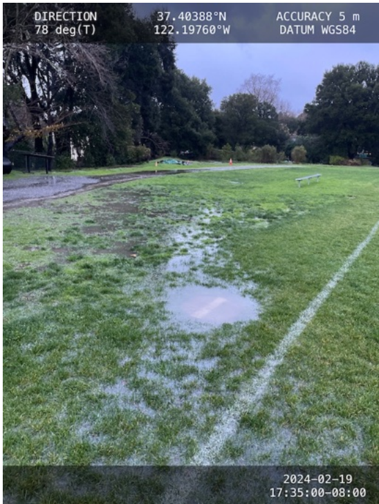
Looking east showing water from field flowing onto fire access road.
