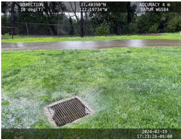
Looking north showing water on access road bypassing field drain
