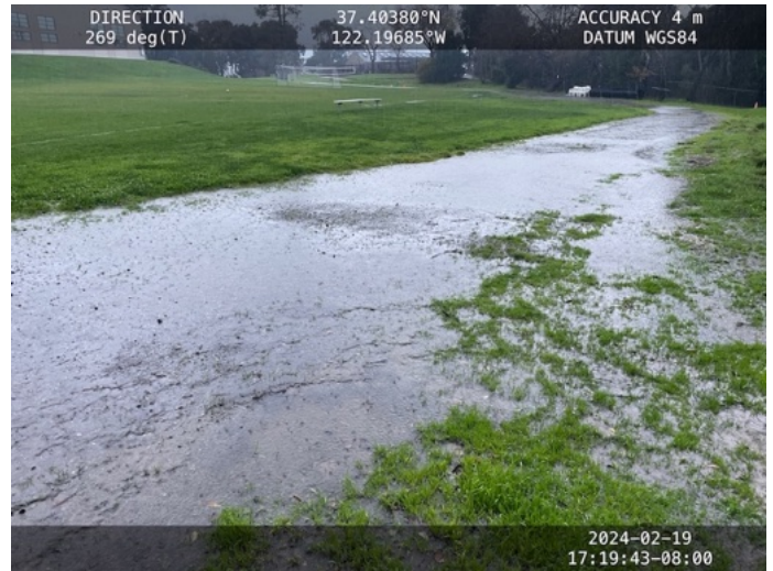
Looking west showing water on access road alongside bioretention basin bypassing both basin and field drain.
