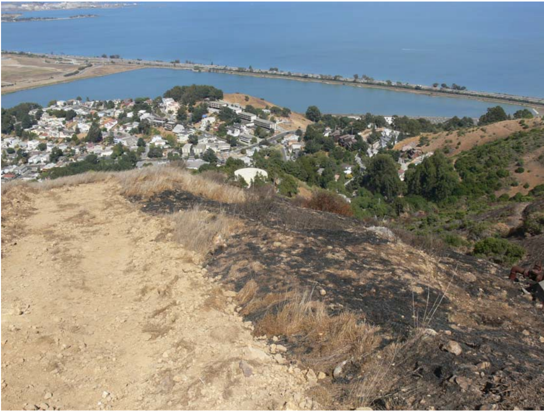
Figure 3. Shallow fire break cut by CDF bulldozer along west side of burn area, along Brisbane Acres Water Tank road. Photo date: 09/20/06.
