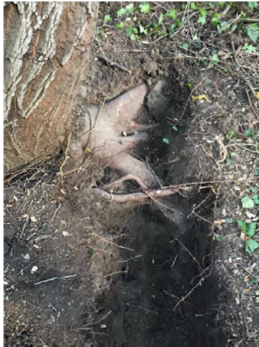
Showing roots that would need to be cut for old lightwell location
